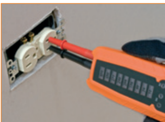
Measure Tamper-Resistant Outlets
