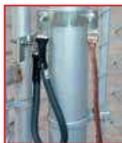
Fence and Gate Jumper Assemblies
