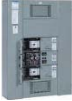
Elevator Control Panelboard
