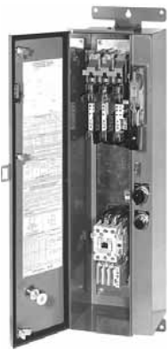
Irrigation Pump Panel—C440 SSOL
