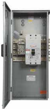
Main Circuit Breaker
