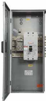
Main Circuit Breaker
