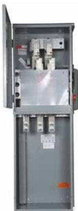
Main Fusible Switch with Utility Pull Box
