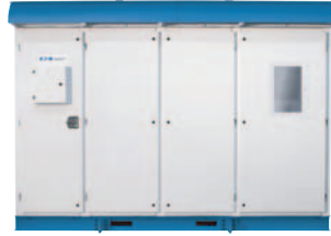
Medium voltage step-up transformer
