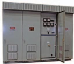
Medium voltage AC switchgear
