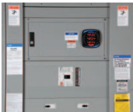
Custom Solar Switchboards
