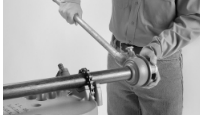
Figure 3 – Sliding Threader On Pipe
