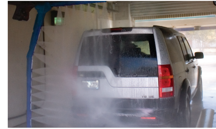
car wash controls
