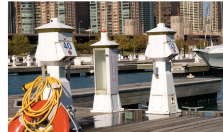
marine shore-power and dock lighting
