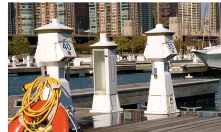
marine shore-power and dock lighting
