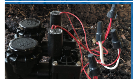
irrigation and sprinkler systems
