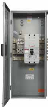
Main Circuit Breaker
