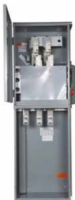
Main Fusible Switch with Utility Pull Box
