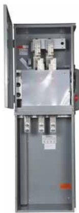
Main Fusible Switch with Utility Pull Box
