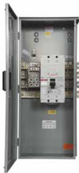
Main Circuit Breaker
